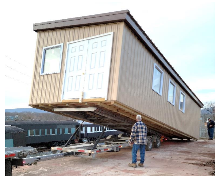
The shell of the new switch tower replica was delivered to the Reading Railroad Heritage Museum on November 29, 2022.
