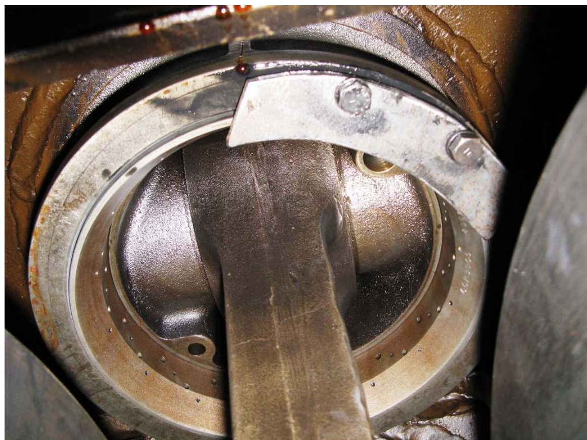
(BOTTOM) Also installed where the pee-pipe had been is the piston blanking plate. This custom-made plate is designed to keep the piston in the liner while allowing the piston pin carrier to pass by after the carrier snap ring has been removed. Leaving the pistons in the liners saved us a lot of time.
